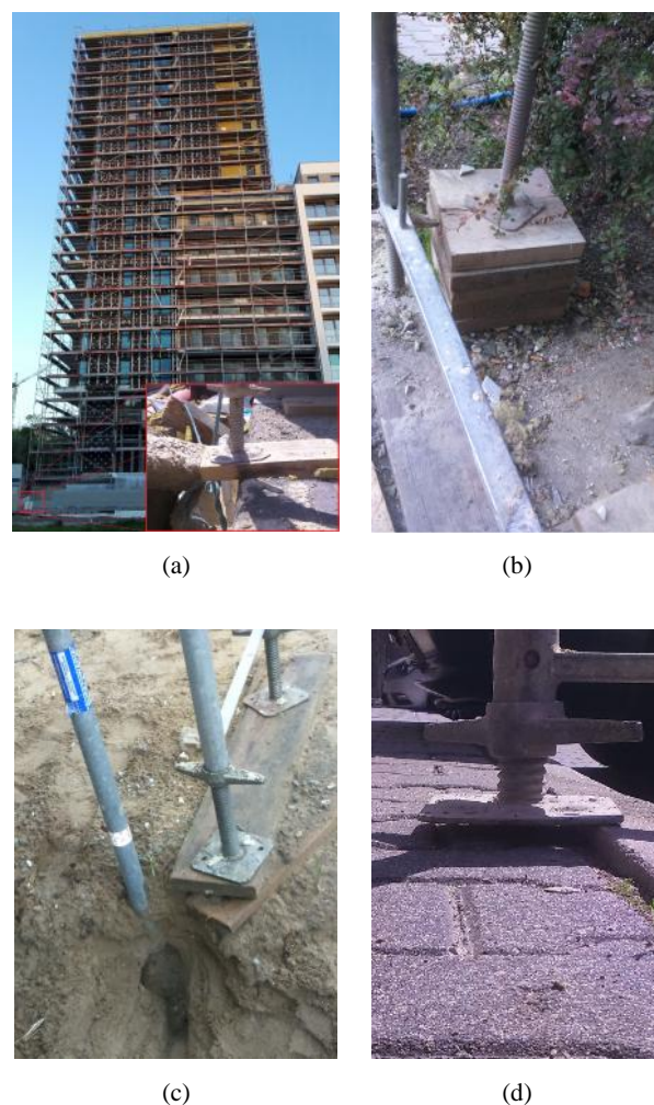
Fig. 2 Errors in scaffolding supports; (a) strained mudsill, (b) multi-level wooden mudsills, (c) unstable substrate, (d) base jack without support
